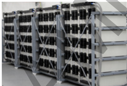
Energy Storage System
